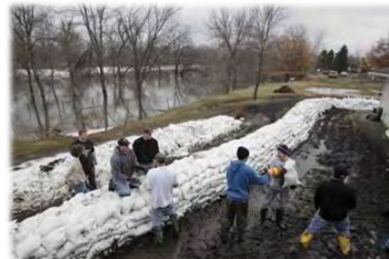
Figure 6: Sandbags are used for flood control (Geiger,O., 2013)
