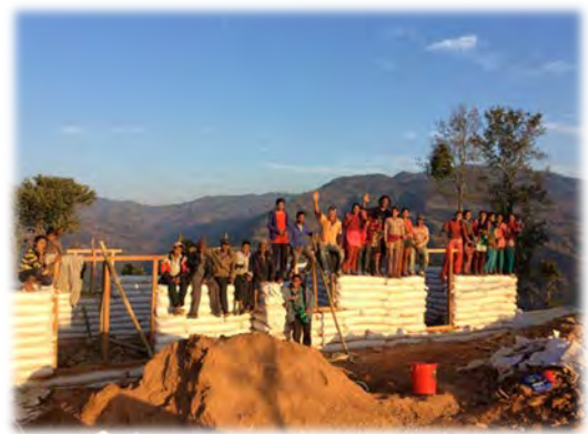
Figure 11: Earthbag School built by First Steps Himalayas survived the earthquake with no damage, Sindhupalchok (Geiger, O., 2013)
